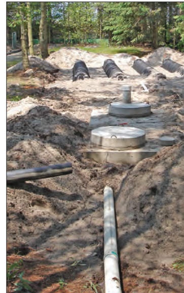
A conventional septic system is installed using chambers on a limited-access site.
