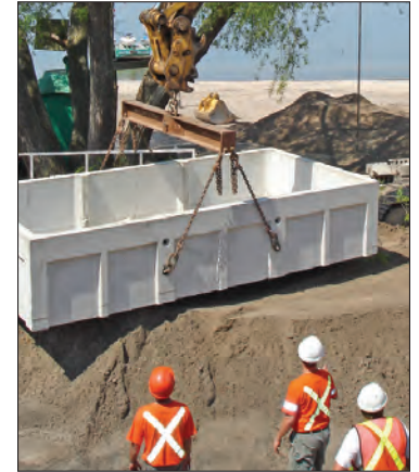
Mike Pauze, Kirk Hastings, and Andy Reid from Brooklin Concrete Products guide a biofilter enclosure into place.
